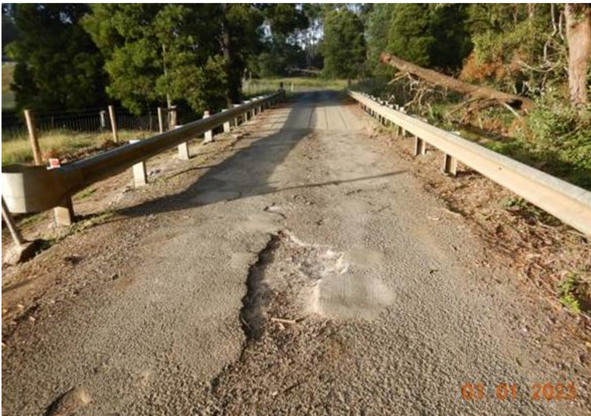
Road surface damage at Burns Road, Wyena
