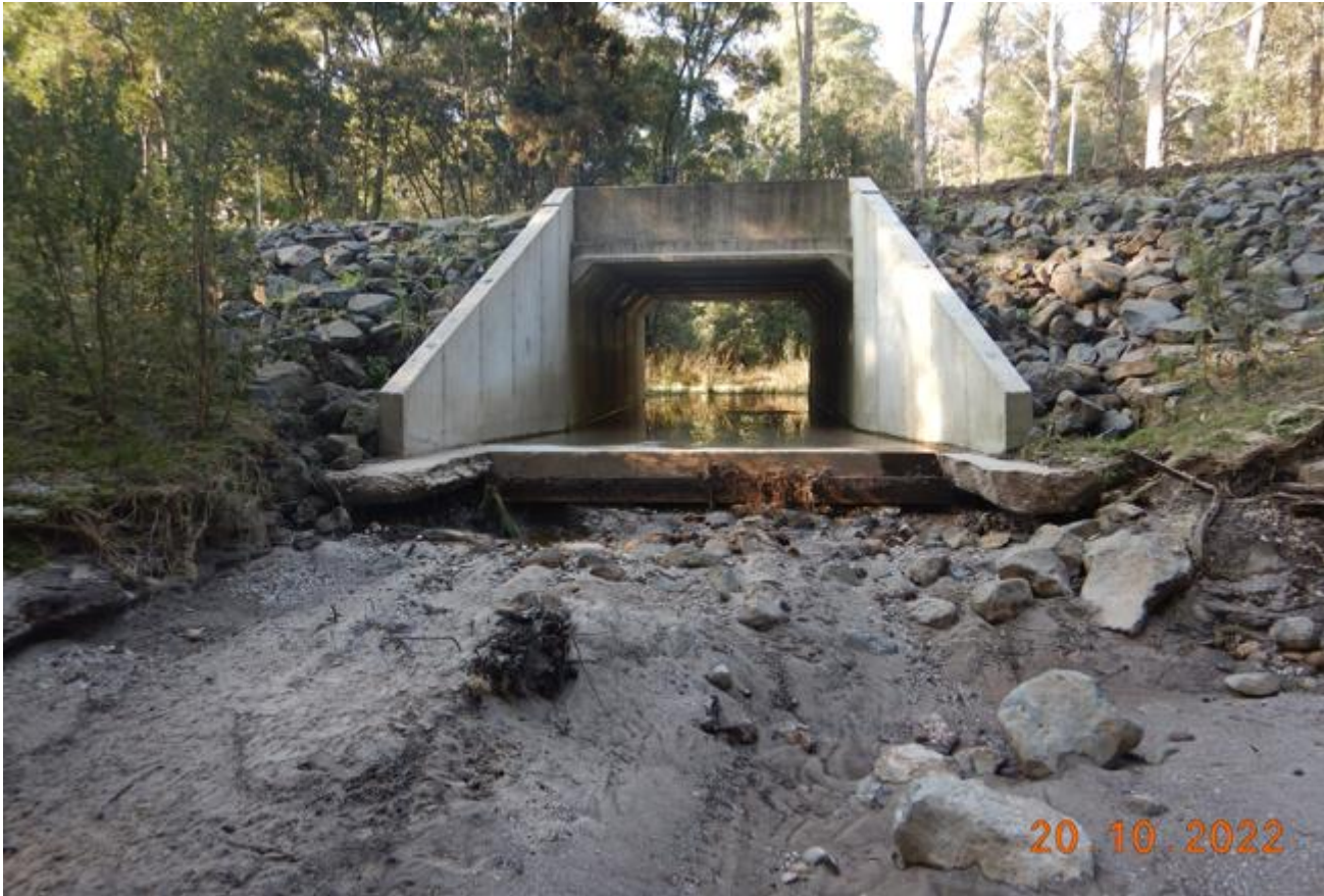
Erosion at Culvert 1527 Banca Road, Winnaleah
