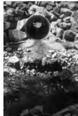
Perched culverts are a barrier to fish passage
