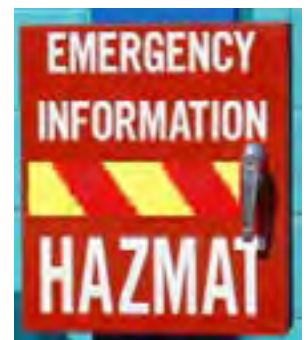
Example of emergency information cabinet
