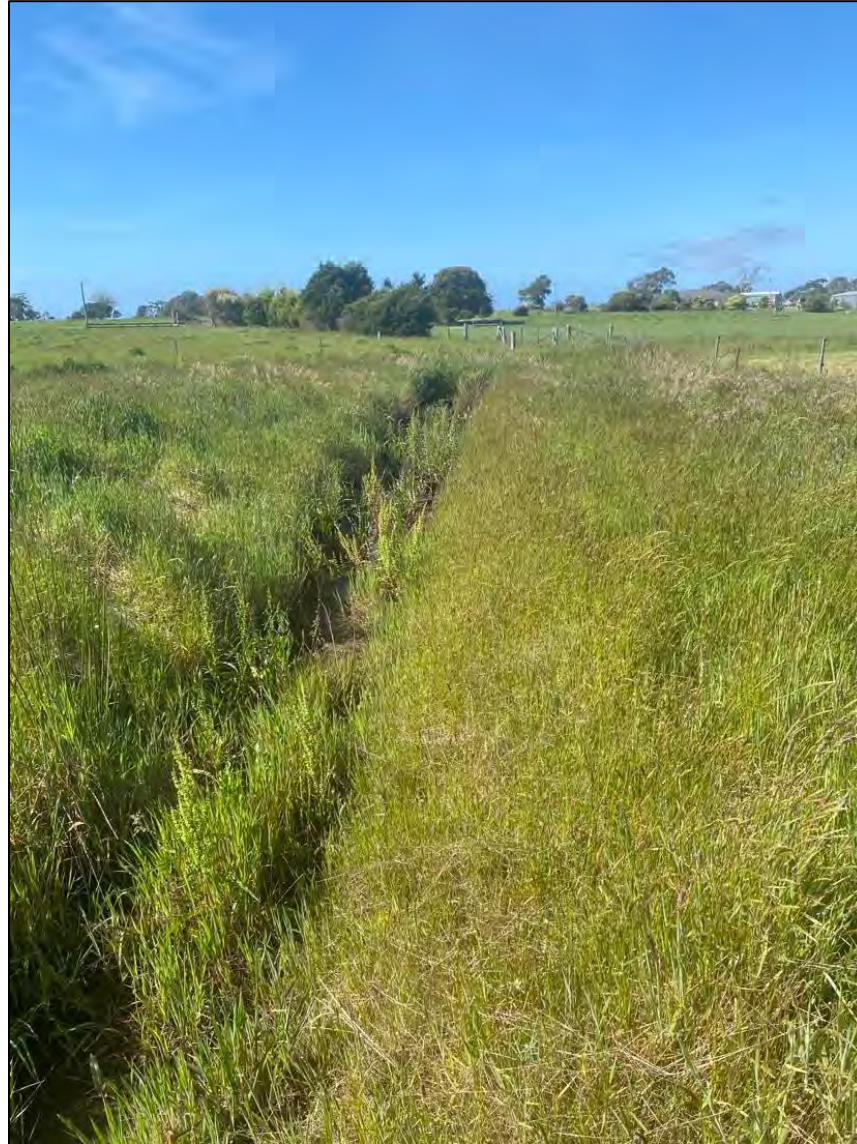
Figure 2 – Existing open drain along eastern boundary of 1954 Bridport Road, facing north towards the north-eastern corner of the subject site (photo taken 9 November 2022).
