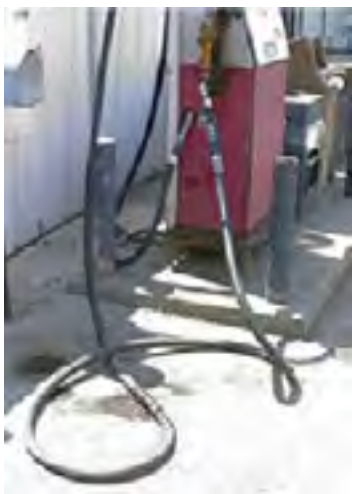
✗ Evidence of leak shown at hose connection
