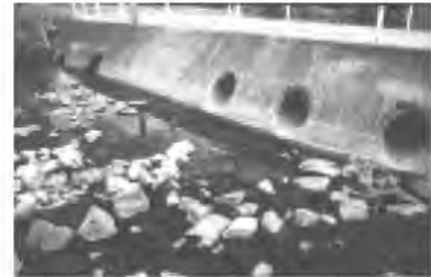
Multi level culverts may allow fish to pass through causeways during low flows
