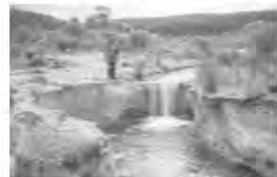
Headcut eroding stream bed
